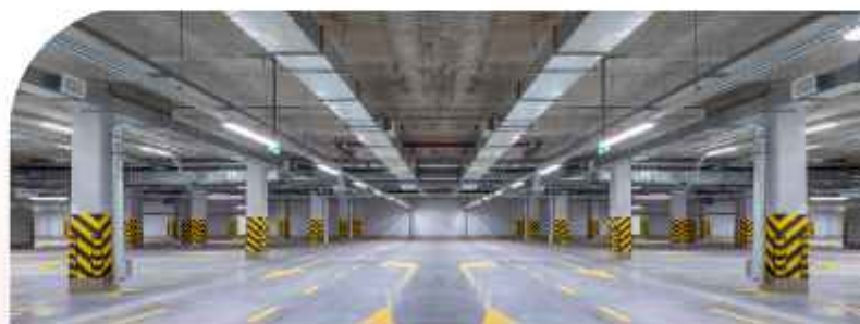
Conventional Ventilation Ducts
